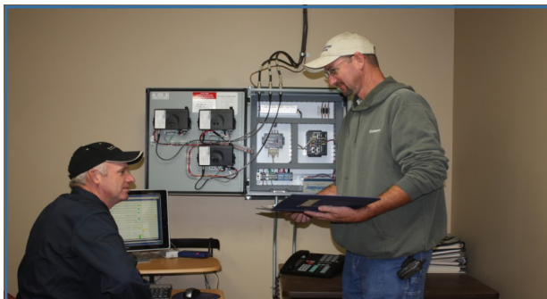
Glenn Garrett & Montie Taylor overseeing the SCADA System
